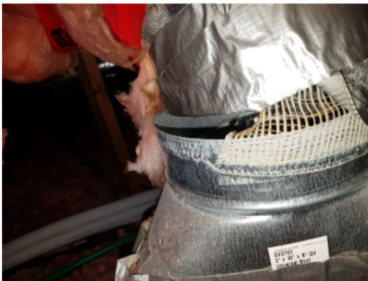
Figure 6 Example of disconnected and leaky ventilation fan ducting (and the ineffectiveness of duct tape for connecting ducts)
