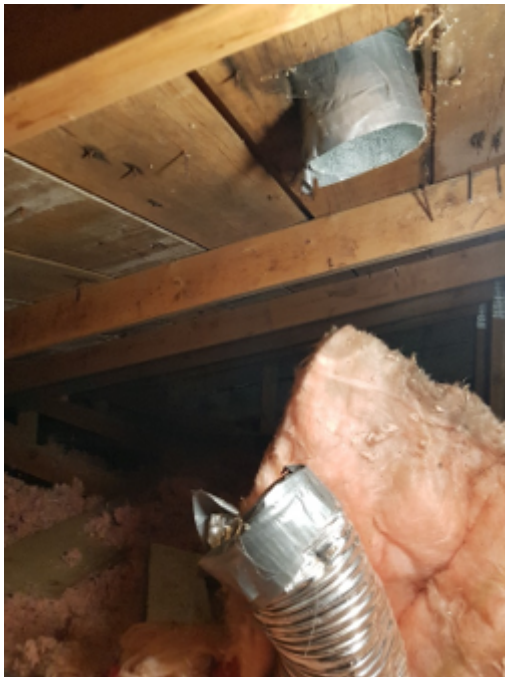
Figure 5 Example of disconnected and leaky ventilation fan ducting (and the ineffectiveness of duct tape for connecting ducts)
