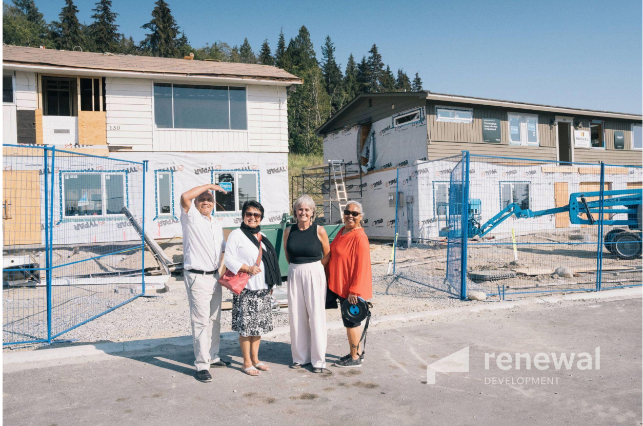
Figure 5: shíshááh Nation Chief and Council in front of the relocated homes under construction.
